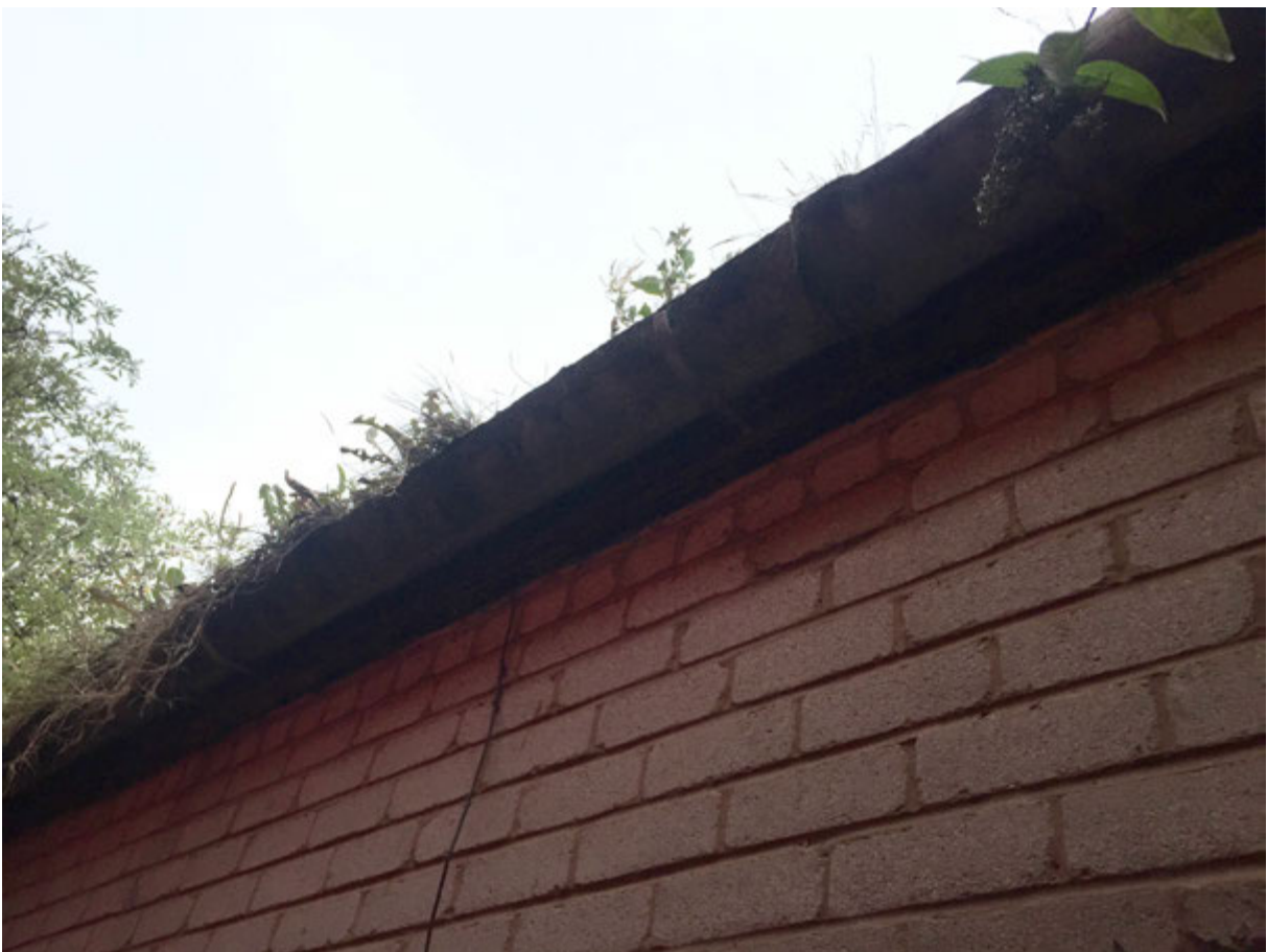
2. Position and condition of rear guttering
